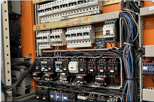
Existing electrical control panel
