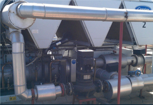
Chilled-water / chiller plant
