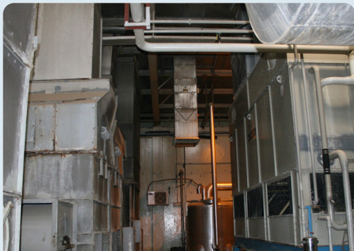
Industrial process cooling utilities
