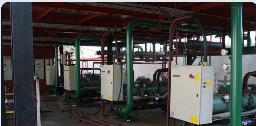
Multi-compressor refrigeration plant
